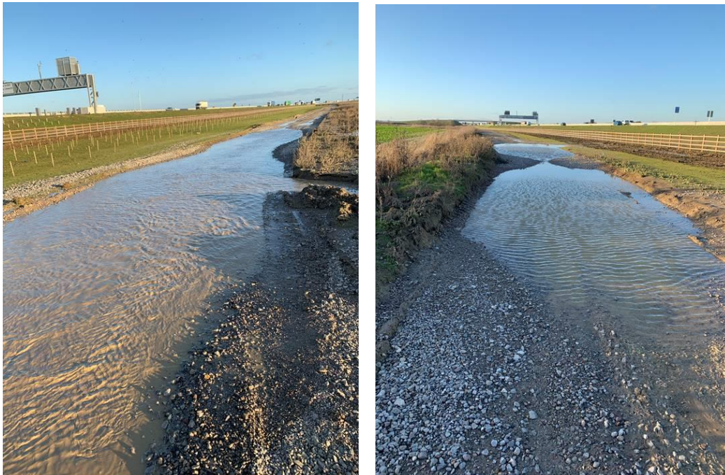
Figure 9 – drainage issues along the A14
